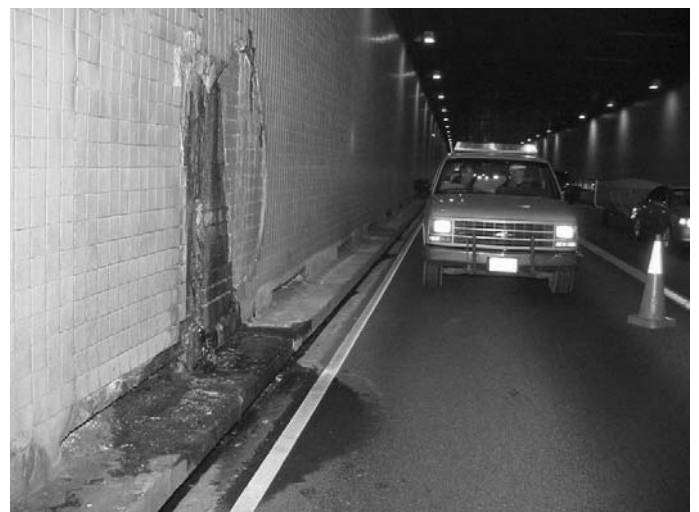
riorated in areas and rebar was exposed, all of which posed a
