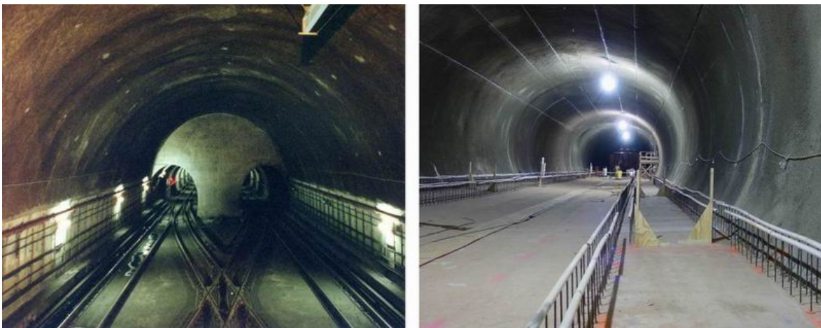
Figure 32a: Shotcrete final lining at Hildarose double crossover WMATA - Wheaton, MD 1985 Figure 32b: Shotcrete final lining at Dulles International Airport pedestrian tunnel - Dulles, VA 2001
