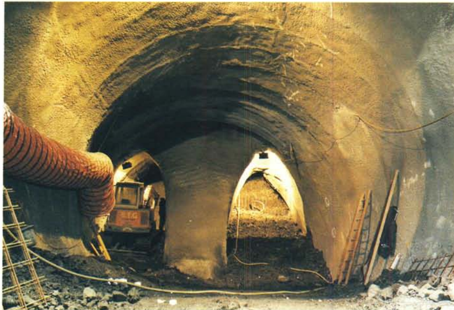
Two side headings in the Type 1 excavation sequence at the Heathrow trial tunnel.
