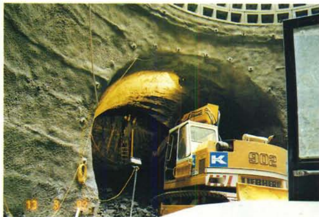
Breakout of the NATM trial tunnel at the bottom of the precast concrete shaft.
