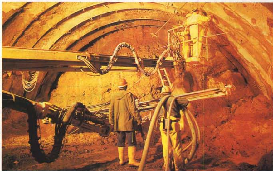
NATM being used in a D-shaped tunnel where reinforced mesh (seen at the top of the final section) is placed prior to arch girders, shotcreting and final rockbolting.
