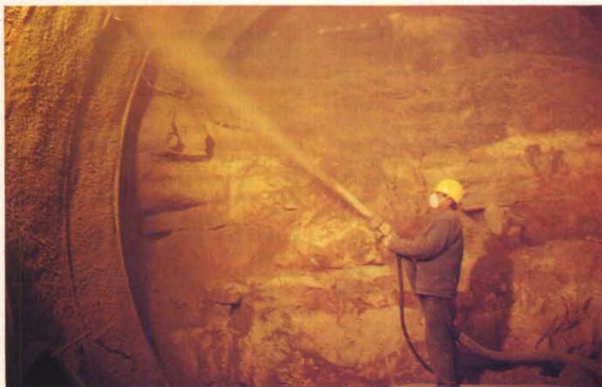
Shotcreting has a rebound of only about 12%, and with the addition of an accelerator the placement of material can be achieved by a skilled operator without reworking.
