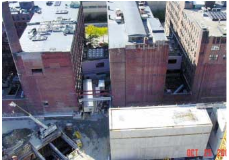
Birds-eye view of the Russia Wharf buildings. One of the construction shafts is seen bottom left
