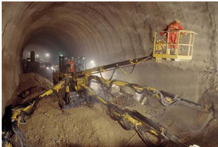
Figure 3: "Boomer" Automated Drill Rig used on the Graz Bypass Tunnel – Graz, Austria 2001
