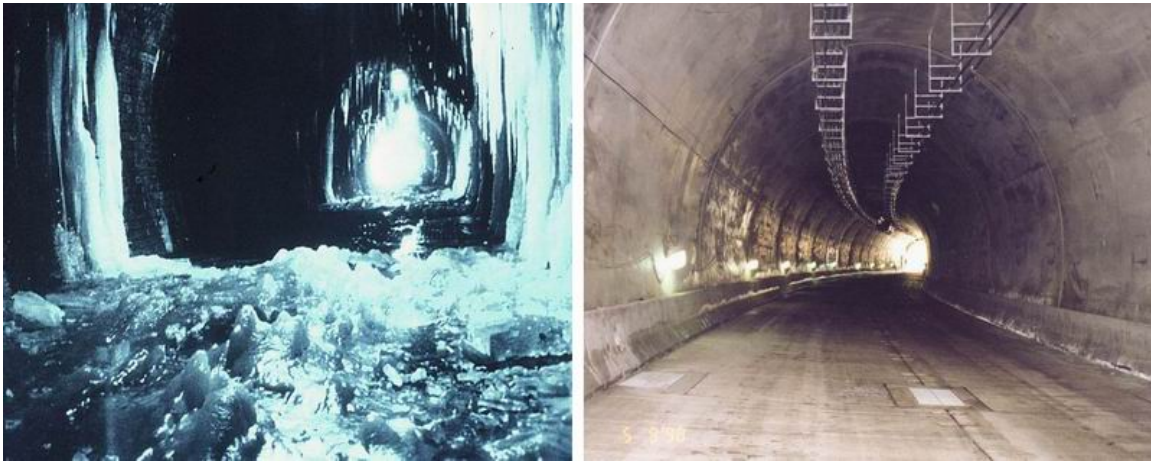
Figure 31a: Berry Street Tunnel prior to rehabilitation - Pittsburgh, PA 1983 Figure 31b: Berry Street Tunnel after rehabilitation – Pittsburgh, PA 1996
