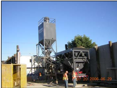
Batch plant inside noise wall at Lander Street gate
